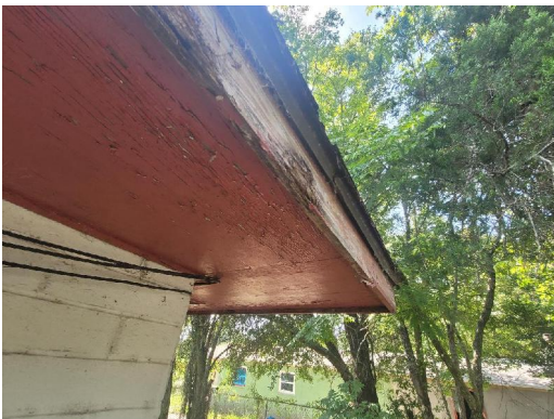
Exterior(001) D-Wall Wood Soffit, Fascia Lead-Positive, Deteriorated (Typical Exterior)
