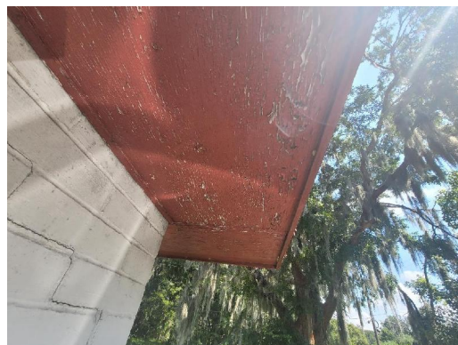
Exterior(001) B-Wall Wood Soffit Lead-Positive, Deteriorated (Typical Exterior)
