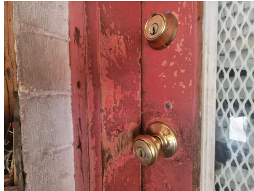
Exterior(001) B-Wall, Right Wood Door Jamb Lead-Positive, Deteriorated
