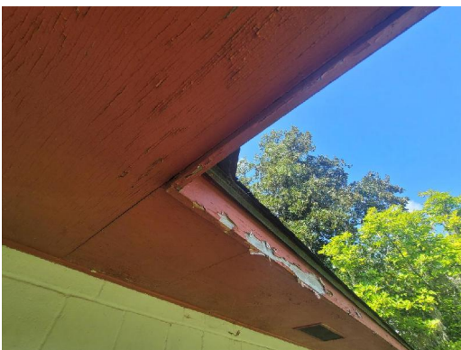
Exterior(001) A-Wall Wood Soffit, Fascia Lead-Positive, Deteriorated (Typical Exterior)
