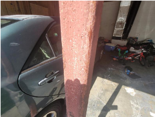
Exterior(001) B-Wall, Right Metal Post Lead-Positive, Deteriorated
